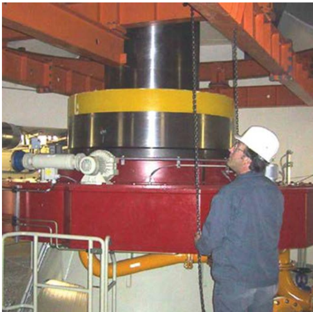
FIGURE 13.9 Shaft between the induction machine and the turbine.
